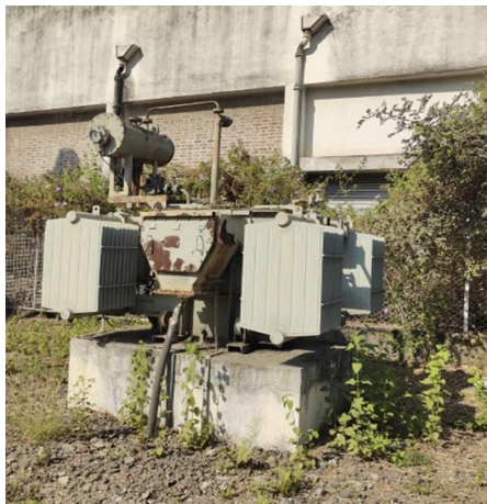
Fig -1: Transformer System
