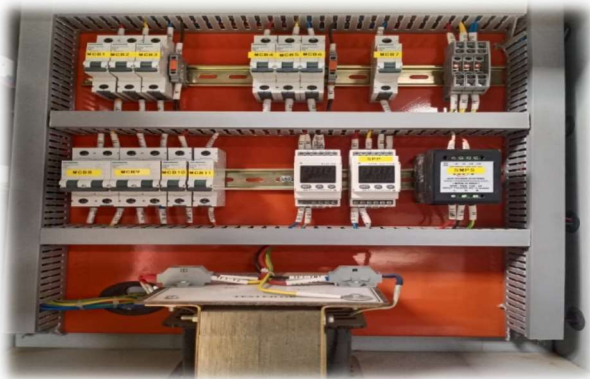
Fig -1: MCC PANEL
